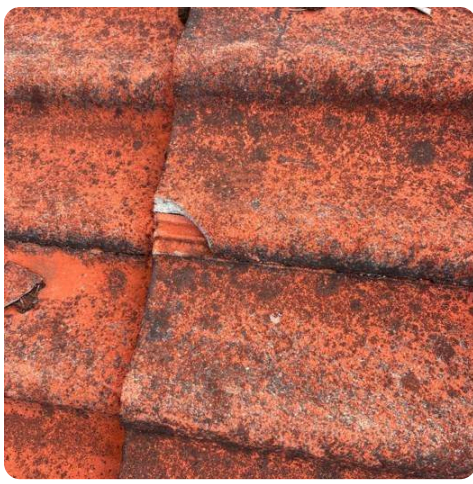
Broken tile with section missing at the side lap, fragment lying on adjacent tile
