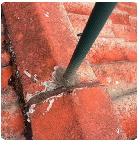
TV antenna mast chased through capping and sealed with silicone only, no Dektite
