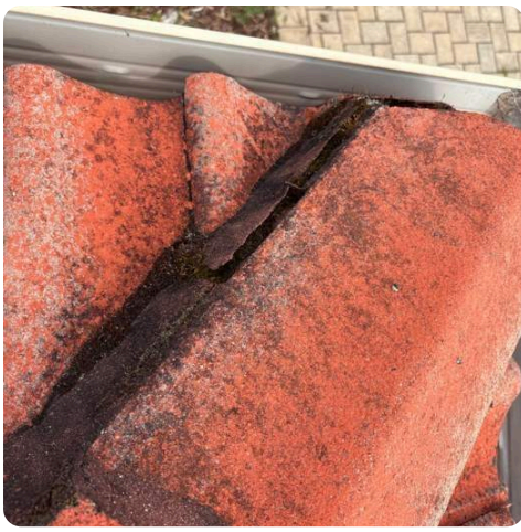
Organic growth held in tile laps at the gutter line
