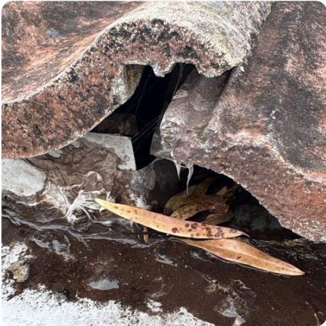
Broken eaves course tile at the gutter line, opening allows water to bypass into the eaves
