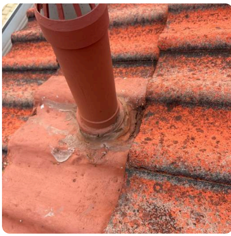
Cracked and deteriorated silicone seal to flue collar and flashing
