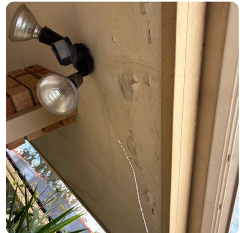
Peeling paint and cracking to eaves lining around sensor light
