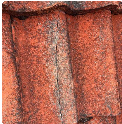
Hairline crack through full length of tile
