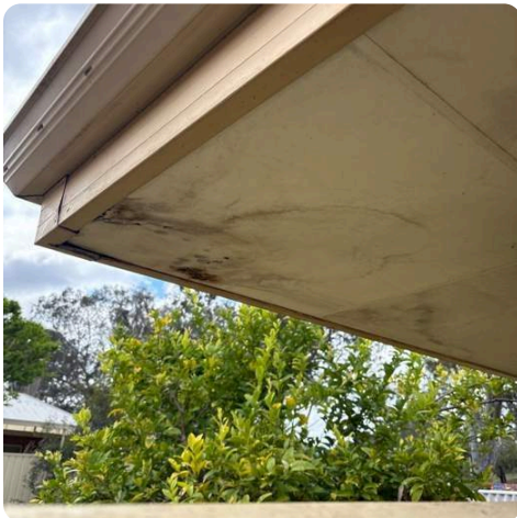
Mould growth and moisture staining to eaves lining at corner consistent with leakage
