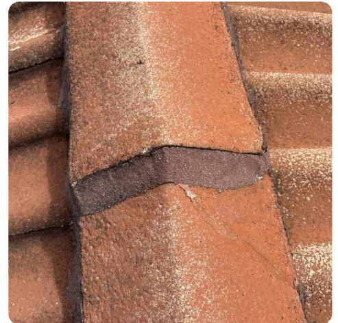
Hairline crack to ridge capping running from the bedding joint
