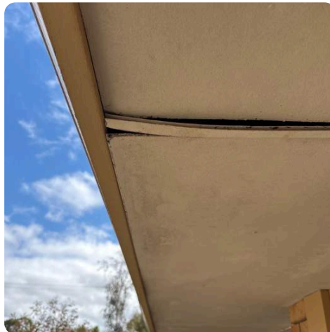
Eaves lining sheet displaced and dropped at the sheet joint adjacent to the fascia
