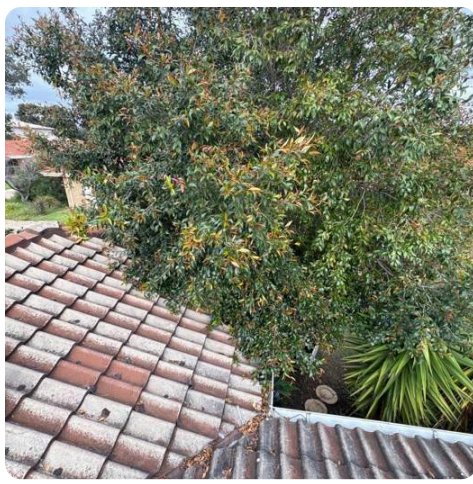
Tree overhanging valley and gutter, debris accumulating
