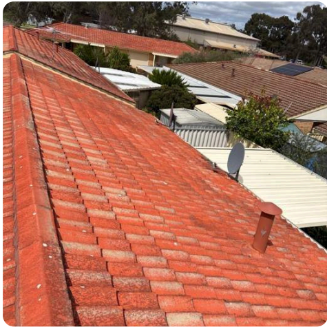
Vent pipe penetration through the tiles with painted cowl
