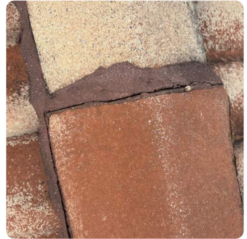
Cracked cement bedding at ridge capping joint, mismatched replacement capping evident
