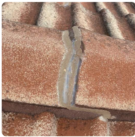
Sealant applied over cracked ridge cap joint
