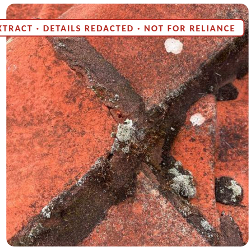
Moss and lichen growth within the ridge capping bedding joint with cracked bedding
