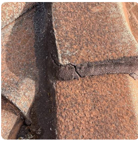
Cracked and separating cement bedding to hip capping
