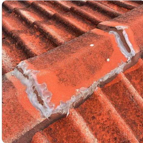
Ridge capping previously sealed with silicone over the bedding joints, sealant weathering
