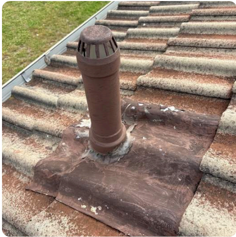
Vent pipe soaker flashing, paint and sealant deteriorating at the collar
