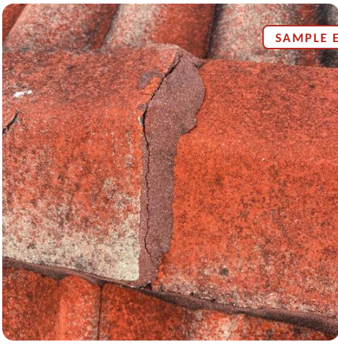
Cracked and separated cement bedding at ridge capping joint
