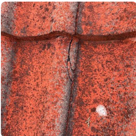
Cracked tile with open fracture running down the pan
