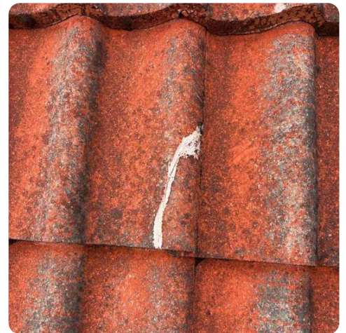
Sealed cracked tile
