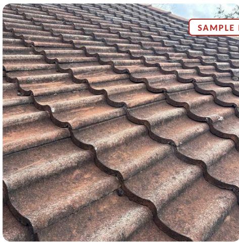
Party wall zone, tiles lifted and misaligned where the wall sits above batten level
