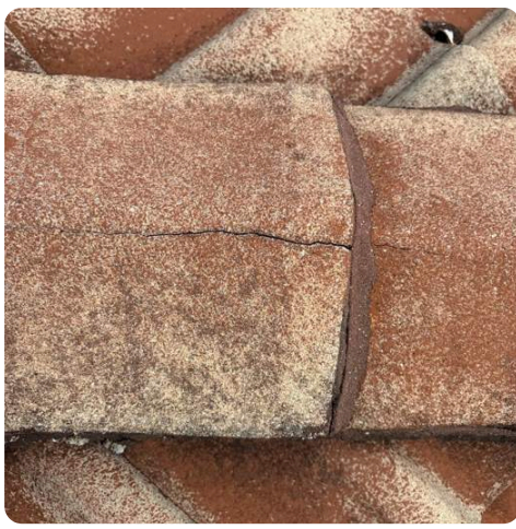
Cracked ridge capping tile
