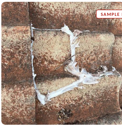
Cracked tile previously silicone sealed, sealant weathered and lifting
