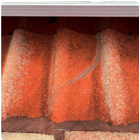
Cracked tile beneath solar panel previously sealed with silicone
