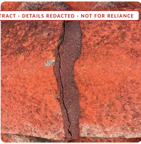
Cracked and lifting cement bedding to ridge capping joint
