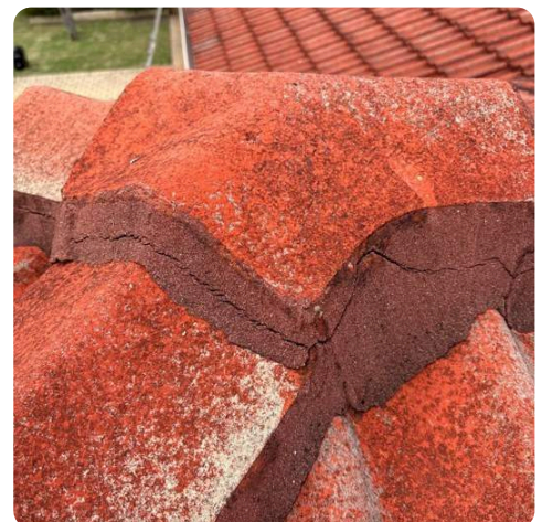
Cracked and separating cement bedding to ridge capping
