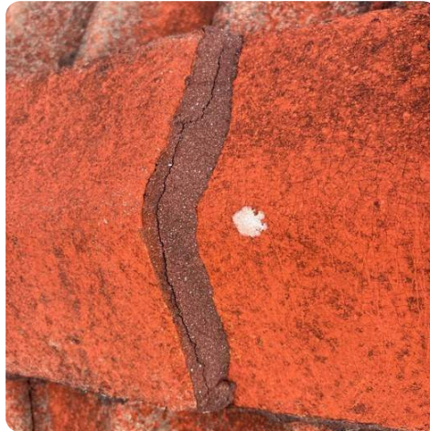
Cracked and separating cement bedding to ridge capping joint
