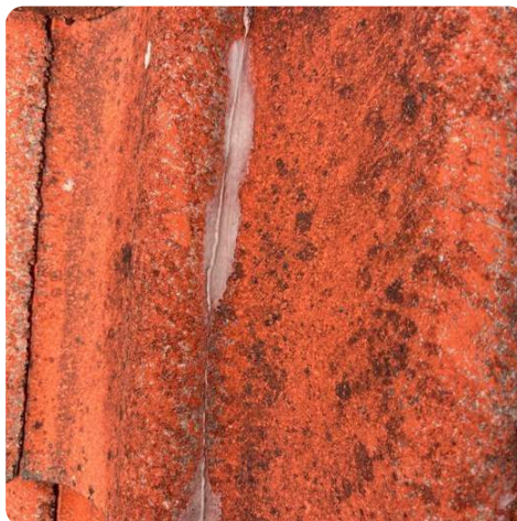
Previously silicone sealed crack to tile, sealant deteriorated and lifting
