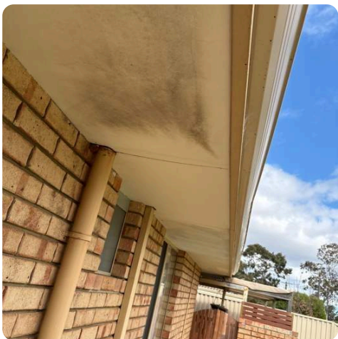
Moisture staining to eaves lining adjacent to downpipe consistent with leakage at the gutter to downpipe connection
