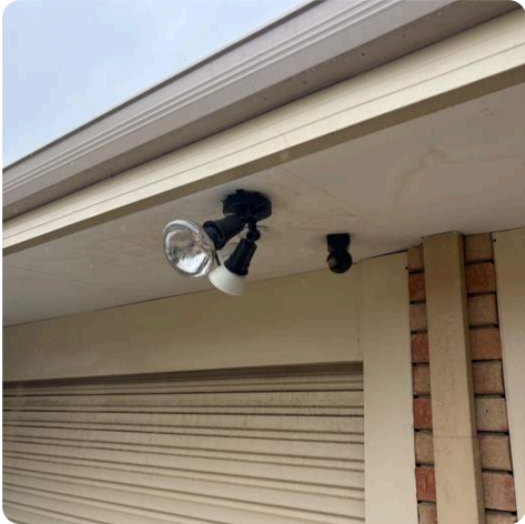
Eaves lining at light fitting, active dripping reported during heavy rainfall
