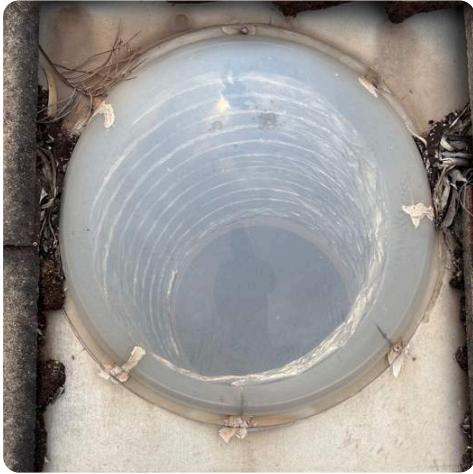
Weathered dome skylight with cracking, sealant repairs at rim and organic matter around flashing
