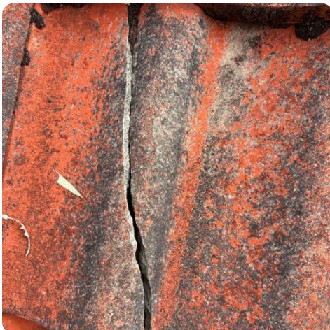
Broken tile with open split
