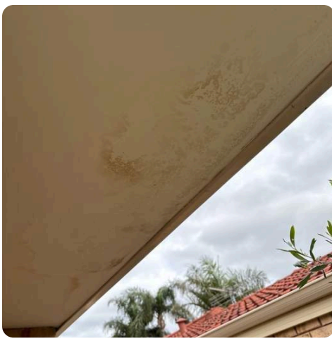
Moisture staining consistent with leakage and blistered paint to eaves lining at gutter edge
