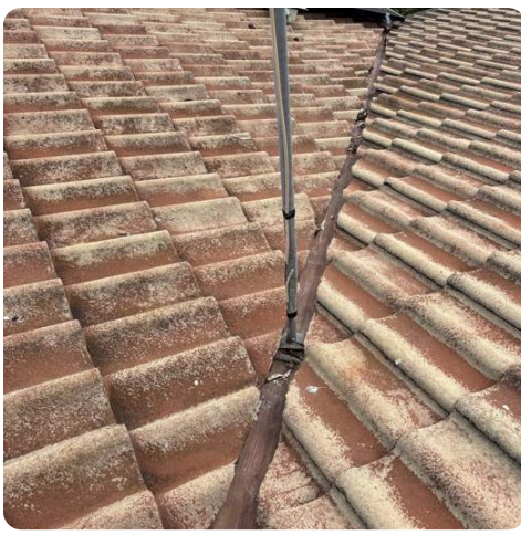
TV antenna mast mounted in valley flashing with cable taped to mast
