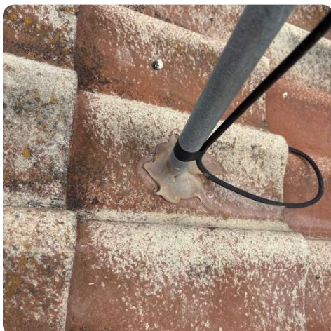
TV antenna mast through tile with sealant only, no Dektite
