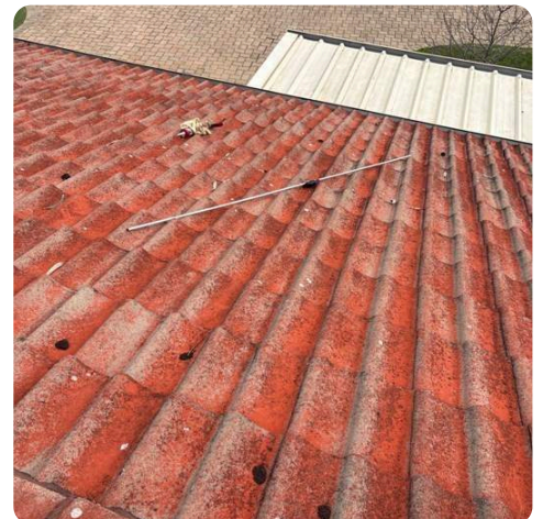
Broken antenna arm lying loose on roof surface
