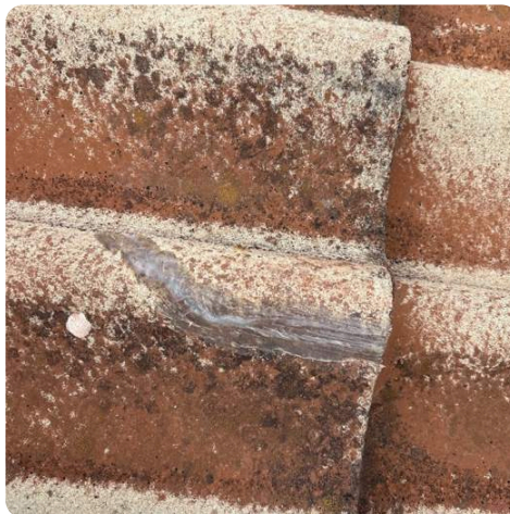
Silicone sealed broken tile
