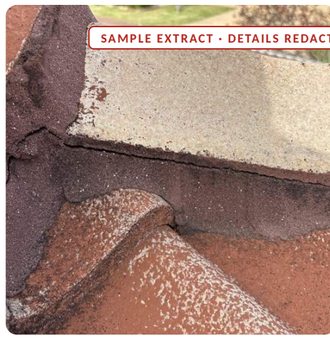
Cracked and eroded cement bedding at the hip and ridge capping junction, capping coating lost
