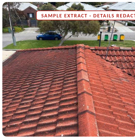
Hip and ridge junction, tiles misaligned adjacent to the right hand hip
