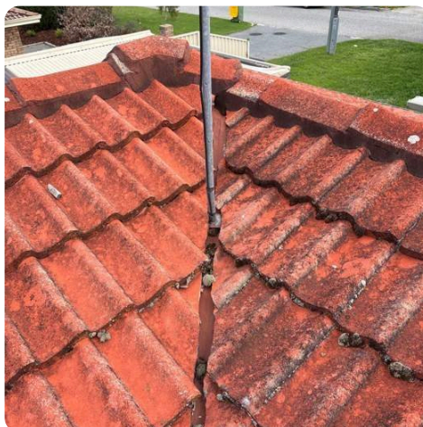
TV antenna mast mounted in the valley flashing, organic matter trapped in the valley
