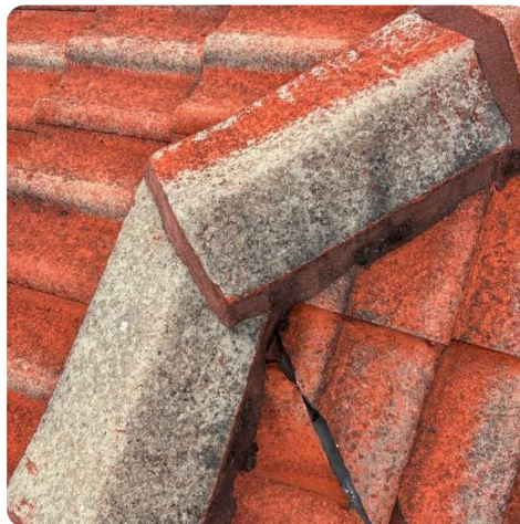
Weathered ridge and hip capping, bedding cracked at apex
