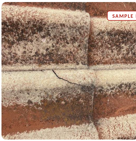
Cracked tile through pan
