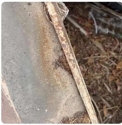
Valley flashing upturn undersized and corroding, organic matter beneath tiles
