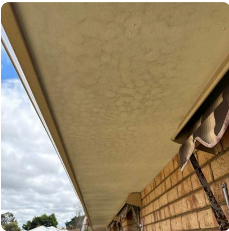
Mottled moisture staining to eaves lining along the gutter line consistent with gutter overflow
