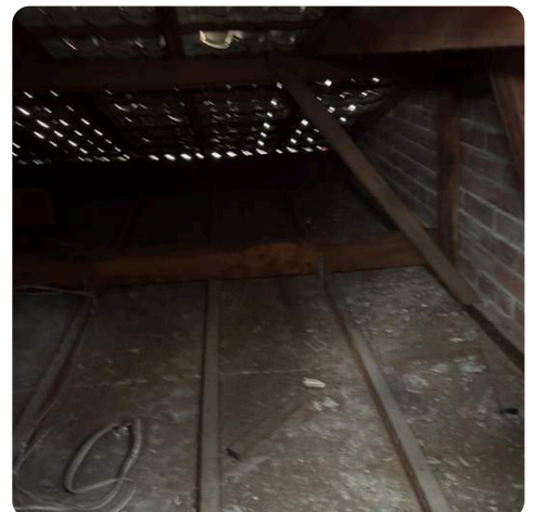
Roof space showing daylight through tile laps, no sarking present
