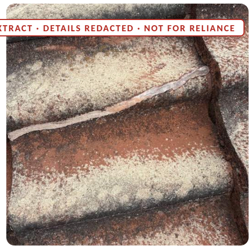
Cracked tile previously silicone sealed across pan
