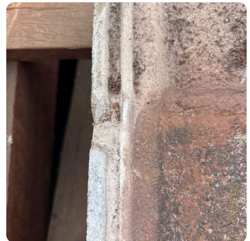
Tile course lifted and misaligned at the party wall line, tile edge sitting proud
