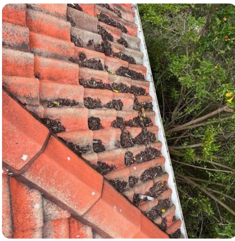
Organic matter build up to tiles at eave edge beneath overhanging vegetation
