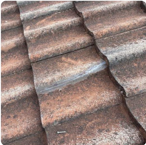
Silicone sealed tile above the living area ingress zone
