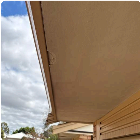
Localised blistering and damage to eaves lining at the fascia edge
