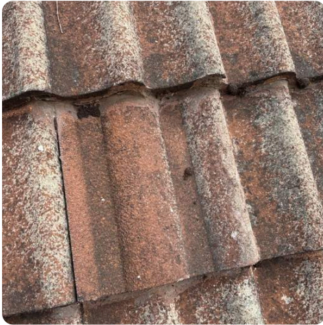
Replacement tile of incorrect profile, gap at head lap packed with mortar
