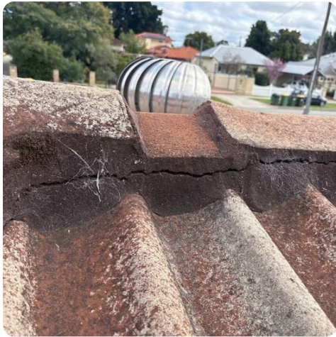
Cracked cement bedding and separated flexible pointing to ridge capping
