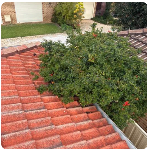
Shrub overhanging gutter at hip corner
