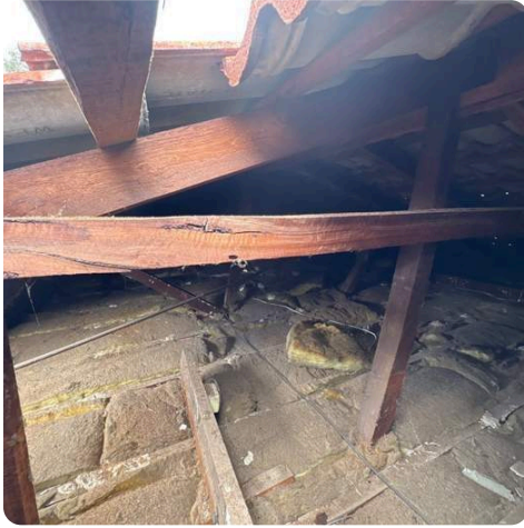
Hardwood under purlin showing a longitudinal check along the grain
