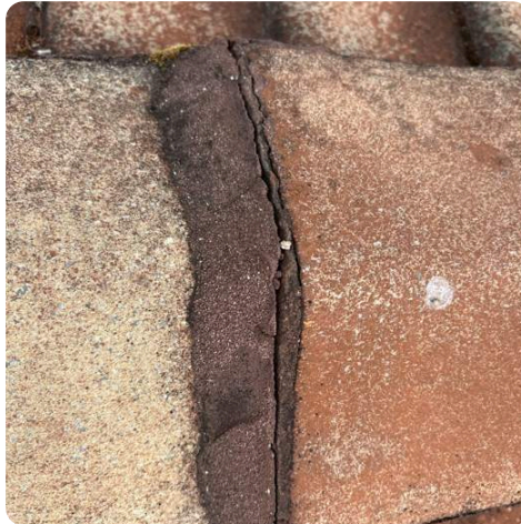
Cracked and separated cement bedding to ridge capping joint
