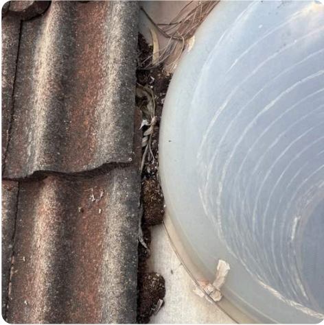
Organic matter packed against skylight flashing beneath tile cuts, restricting drainage
