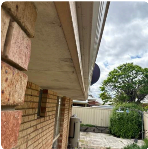
Moisture staining to eaves lining consistent with leakage from gutter overflow
