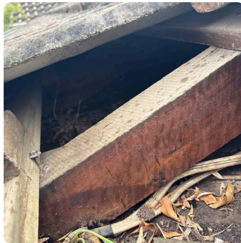
Eaves cavity, moisture staining to rafter consistent with leakage
