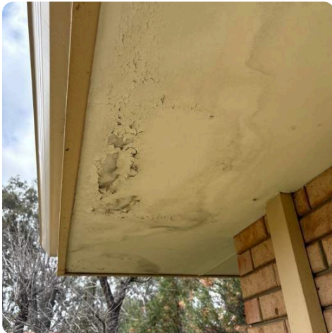
Paint peeling and moisture staining to eaves lining consistent with leakage
