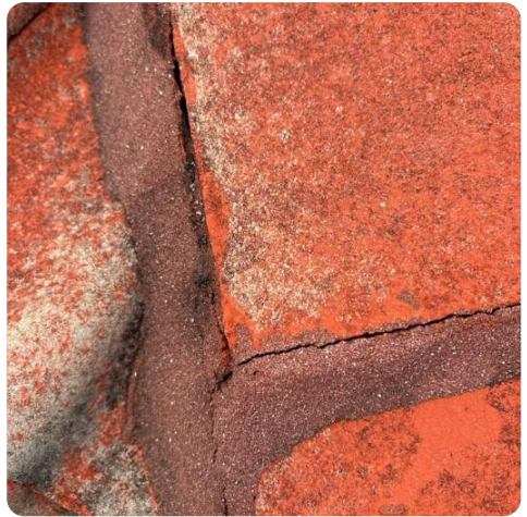
Cracked bedding at hip and ridge junction with coating breakdown
