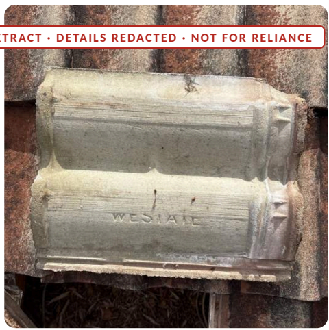
Tile underside showing moisture on the tile body, consistent with moisture retention, no sarking beneath
