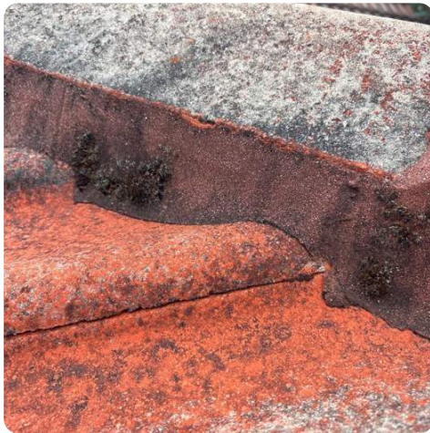
Organic growth to cement bedding beneath ridge capping
