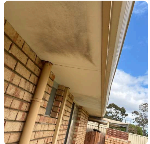
Moisture staining to eaves lining adjacent to downpipe consistent with leakage at the gutter to downpipe connection
