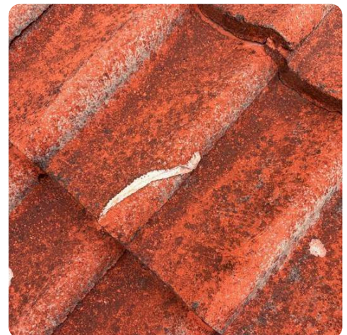
Cracked tile previously repaired with silicone sealant
