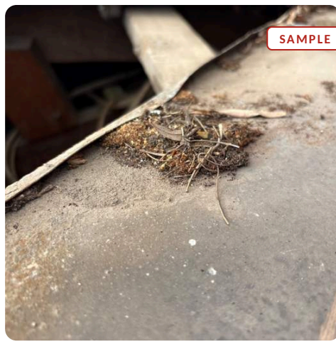
Valley upturn flattened, organic matter build up in valley
