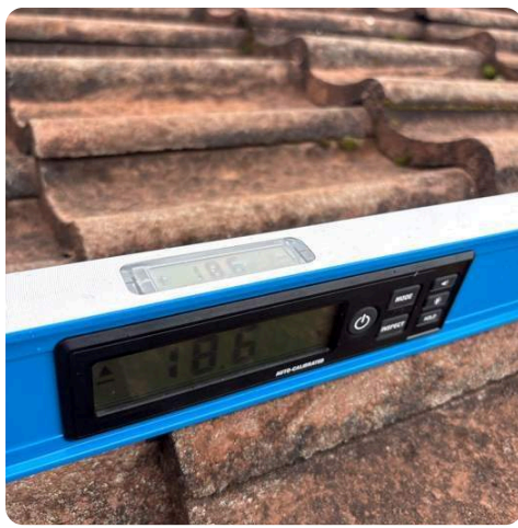
Roof pitch reading, approximately 18.6 degrees at 1x test location
