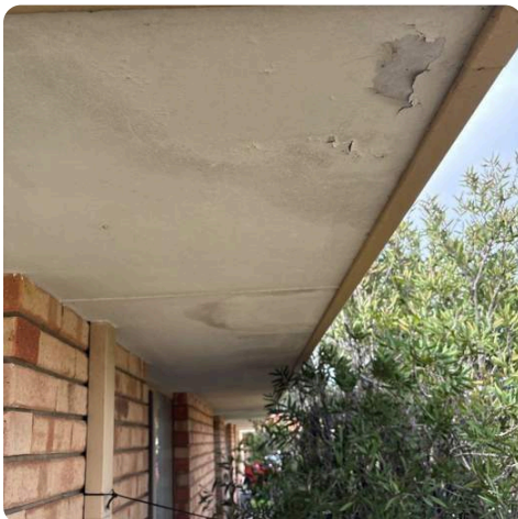
Paint blistering and moisture staining to eaves lining at the hip end corner consistent with leakage
