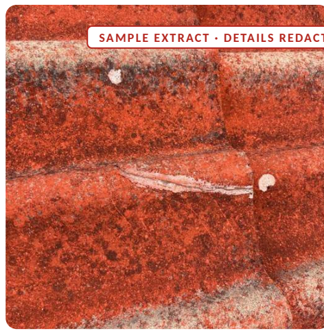
Chipped tile nose exposing substrate
