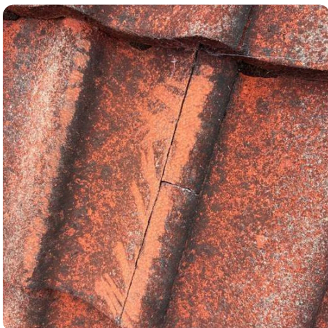
Cracked tile, crack running the full length of the tile
