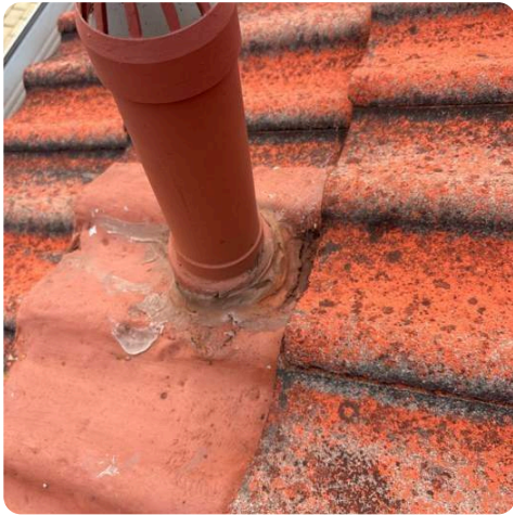
Cracked and deteriorated silicone seal to flue collar and flashing
