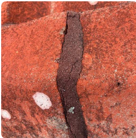
Cracked and eroded cement bedding at the ridge capping joint
