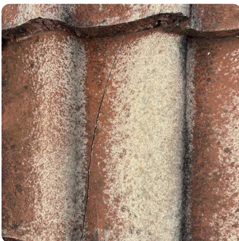
Hairline crack through full length of tile
