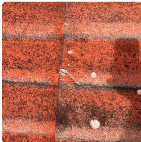
Broken tile corner at the side lap with exposed substrate
