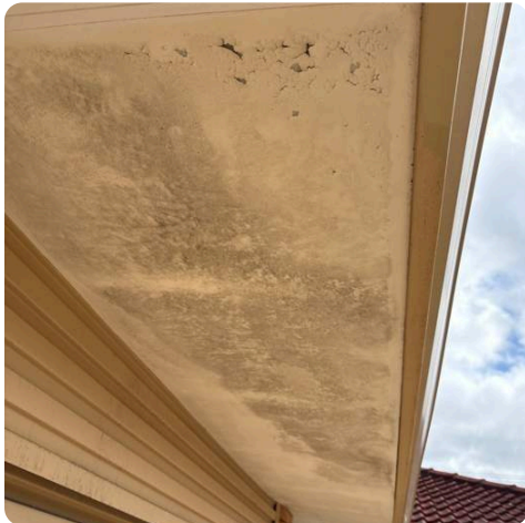
Moisture staining and peeling paint to eaves lining consistent with leakage
