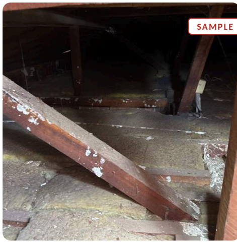
Roof space showing strut and ceiling framing with droppings on timbers
