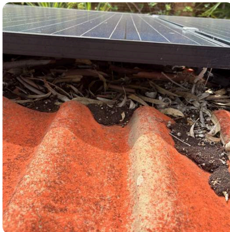
Organic matter build up beneath solar array
