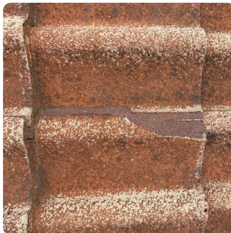
Broken tile, section of lower edge missing exposing the tile below
