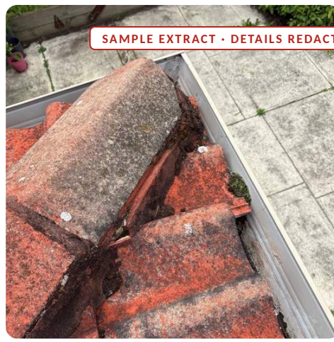
Cracked bedding and moss growth to hip capping end at gutter corner
