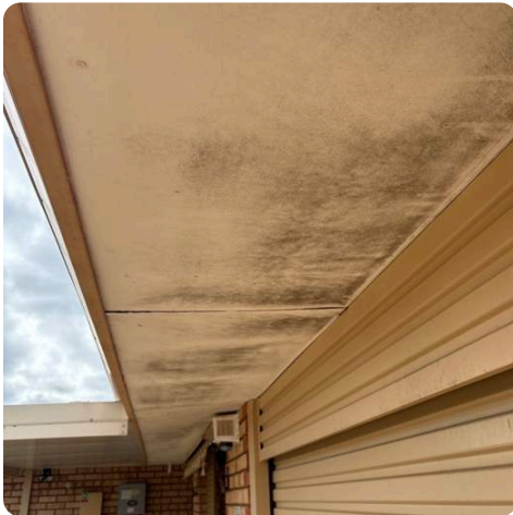
Mould growth and moisture staining to eaves lining above garage consistent with leakage
