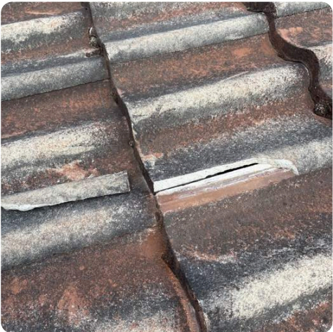
Broken tile with displaced fragment, opening to the tile below
