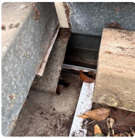
Gutter to downpipe connection, corrosion and debris, suspected leak point into the eaves
