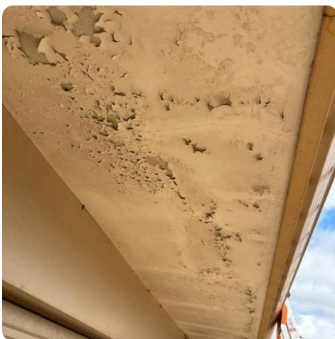
Peeling and blistered paint to eaves lining adjacent to garage, consistent with repeated moisture exposure
