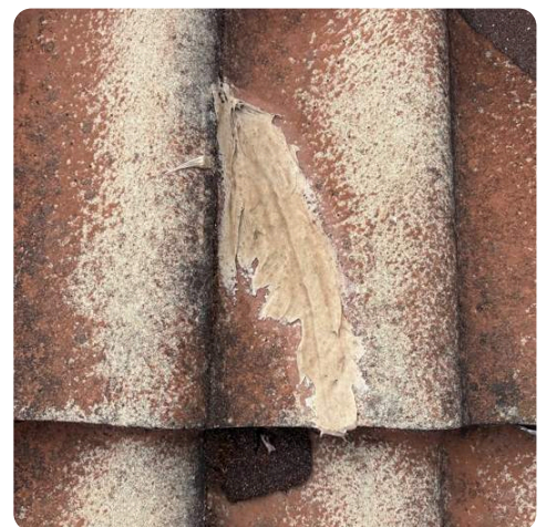
Broken tile previously patched with mortar, temporary repair only
