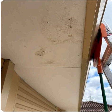
Blistered and peeling paint with moisture staining to eaves lining adjacent to garage
