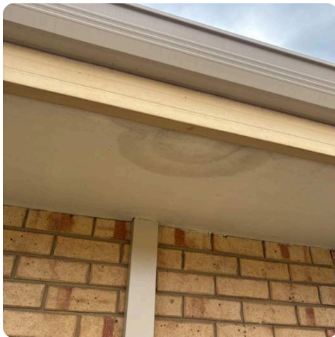
Eaves lining at downpipe, moisture staining consistent with leakage at the gutter connection
