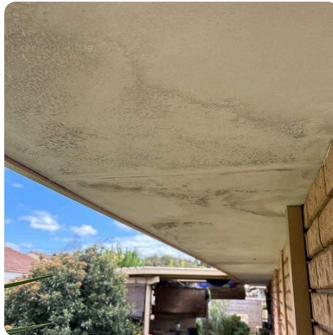
Moisture staining across eaves lining consistent with leakage from the internal downpipe elbow
