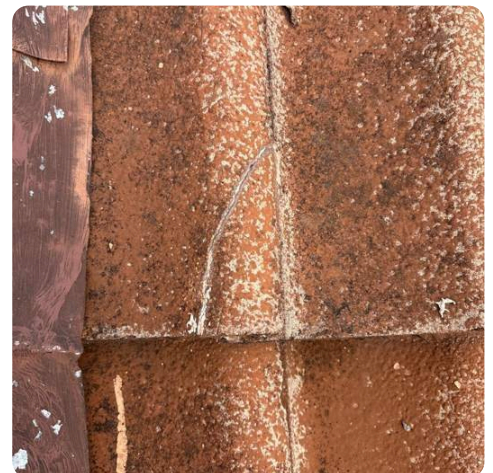
Silicone sealed crack to tile adjacent to the valley flashing
