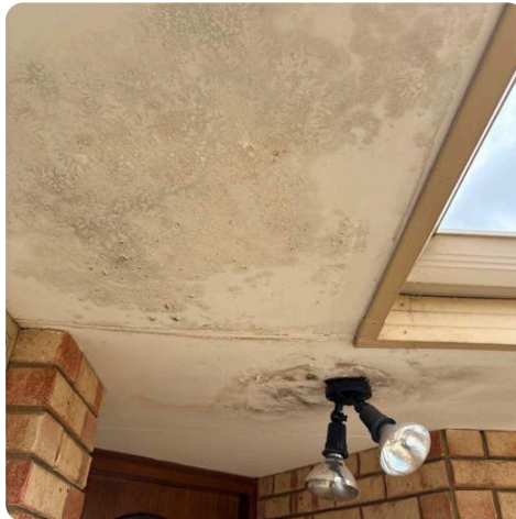
Peeling paint and mould growth to porch lining, moisture staining around light fitting
