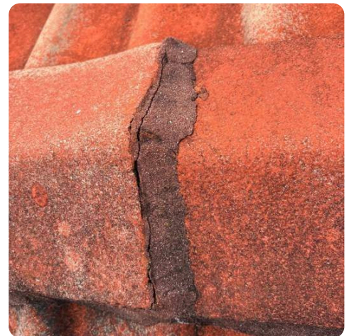
Cracked and separating cement bedding to ridge capping joint
