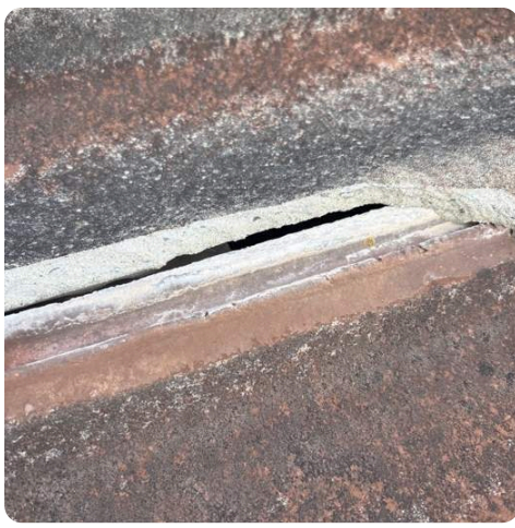
Cracked tile with lap lifted, open gap into the roof space
