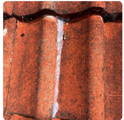
Cracked tile previously sealed with silicone, temporary repair only
