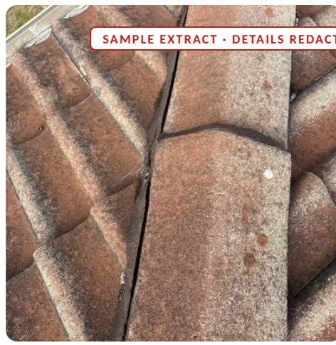
Eroded cement bedding and cracked pointing along hip capping
