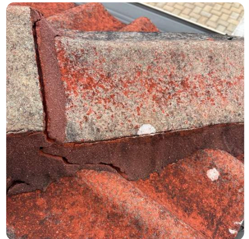
Cement bedding cracked and separated beneath hip capping
