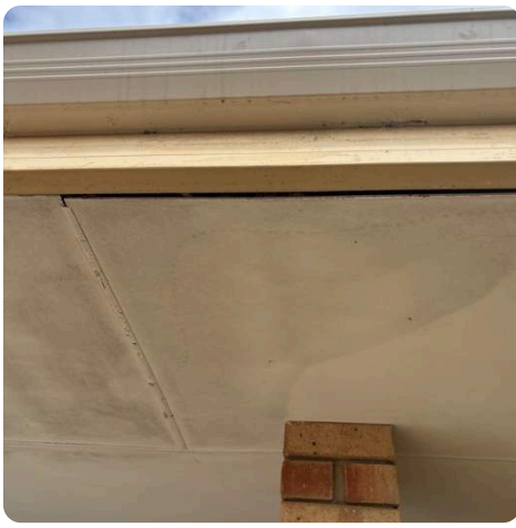
Eaves lining displaced at the fascia line with an open gap and moisture staining
