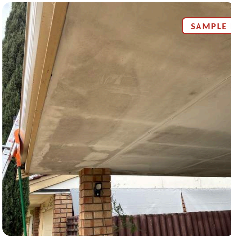
Moisture staining across eaves lining consistent with leakage
