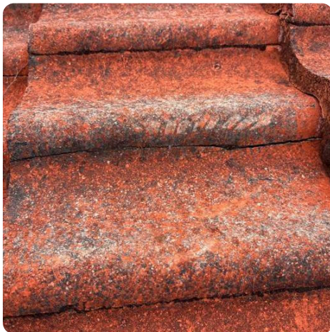
Cracked and spalling tile nose
