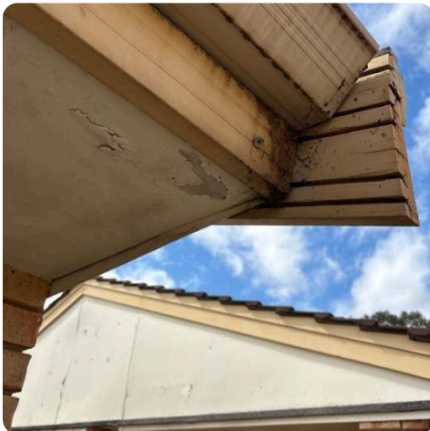
Eaves corner with paint flaking and moisture staining to fascia and eaves lining consistent with leakage from the gutter above
