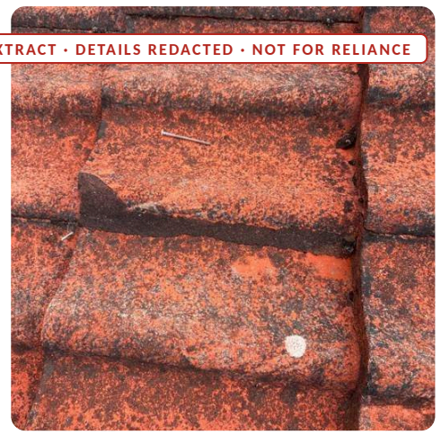
Loose roofing nail on tile surface, adjacent tile with chipped lower edge
