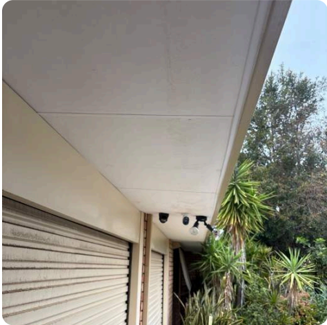
Front eaves lining, moisture staining consistent with leakage across sheet joints
