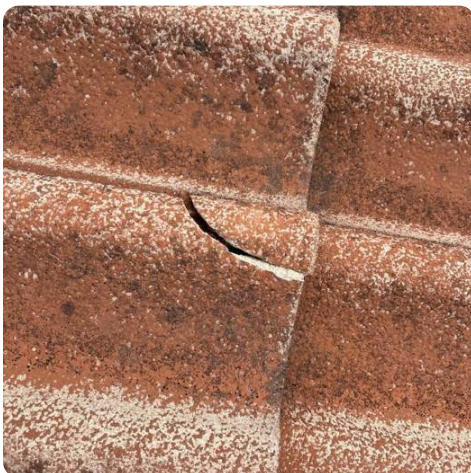
Cracked tile with broken section lifted at the side lap
