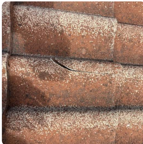
Cracked tile with open fracture across the pan
