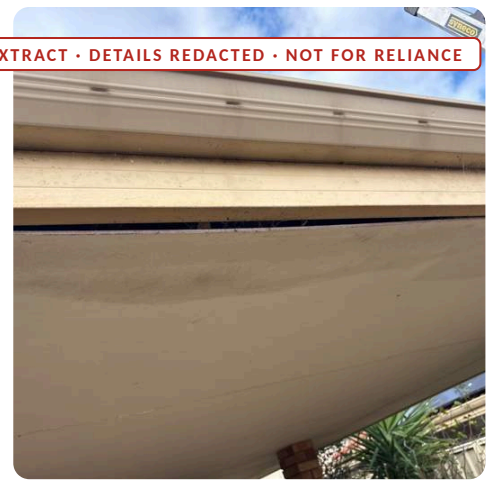
Eaves lining separated from fascia trim leaving open gap
