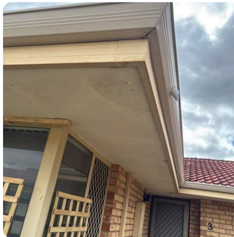
Eaves lining at gutter mitre, moisture staining consistent with leakage
