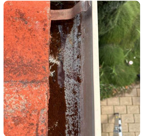
Gutter holding standing water and sediment, indicating inadequate fall toward the outlet
