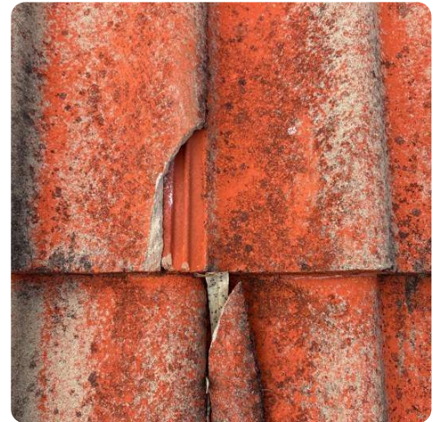
Broken tile with fragment lying on course below
