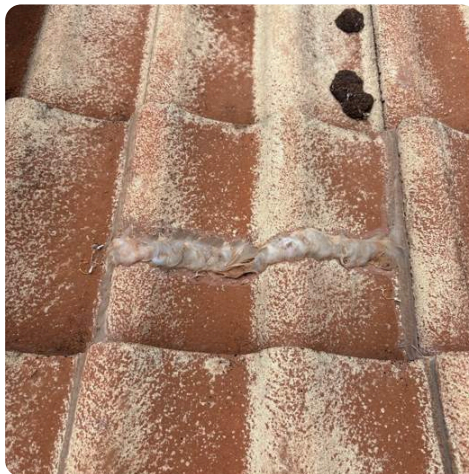
Cracked tile previously silicone sealed across pan, sealant weathered
