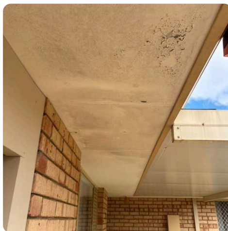
Moisture staining consistent with leakage and blistered paint to eaves lining at front entry
