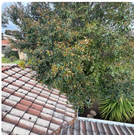
Tree overhanging valley and gutter, debris accumulating
