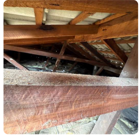
Roof framing showing a rafter with a large knot and a lapped pine section fixed alongside
