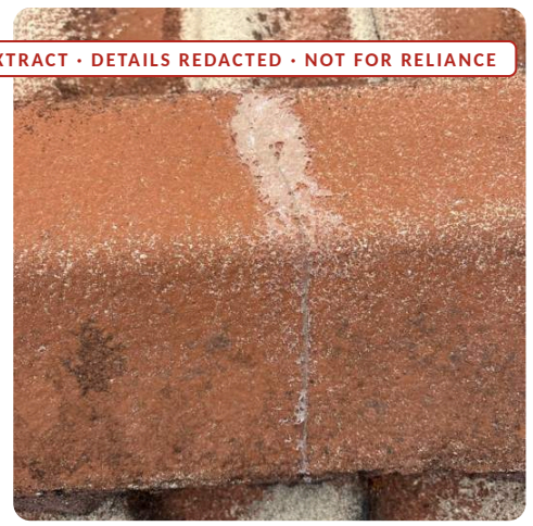
Cracked ridge cap with historic silicone repair
